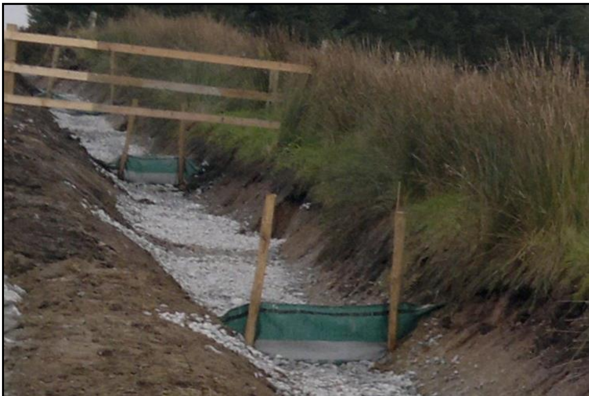
Figure 46: Example of a silt fence used in conjunction with check dams along roadside drainage channels
