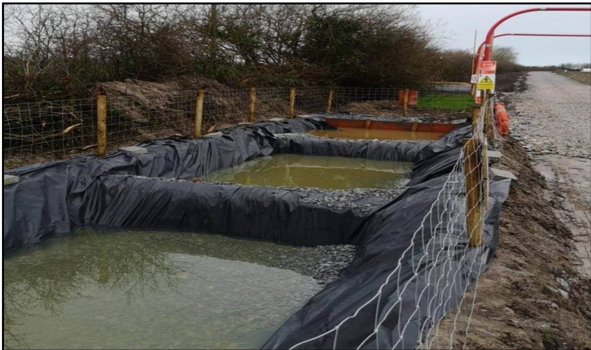
Figure 44: Multi-tiered settlement pond with stone filter
