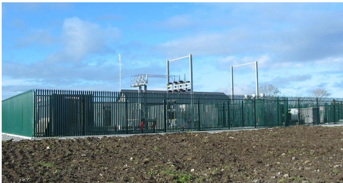
Figure 30: Typical Substation Compound
