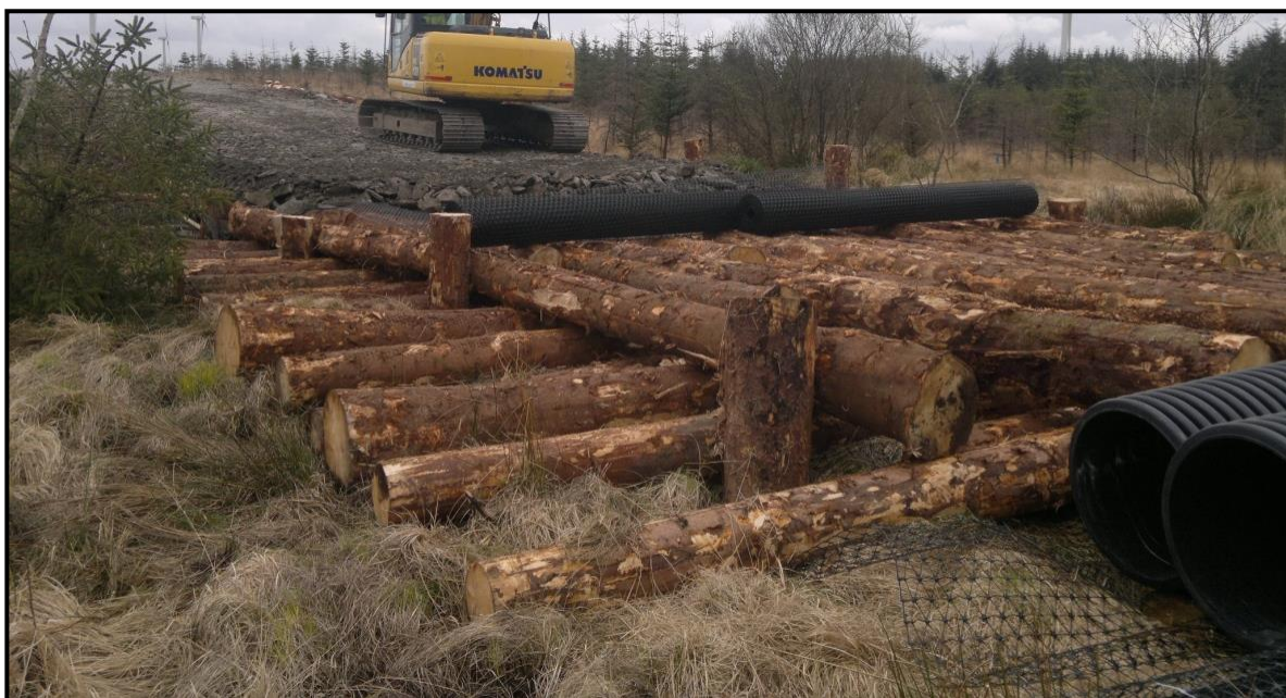
Figure 4.5 Option 2 -Typical floated road using Timber Log Construction on a wind farm
