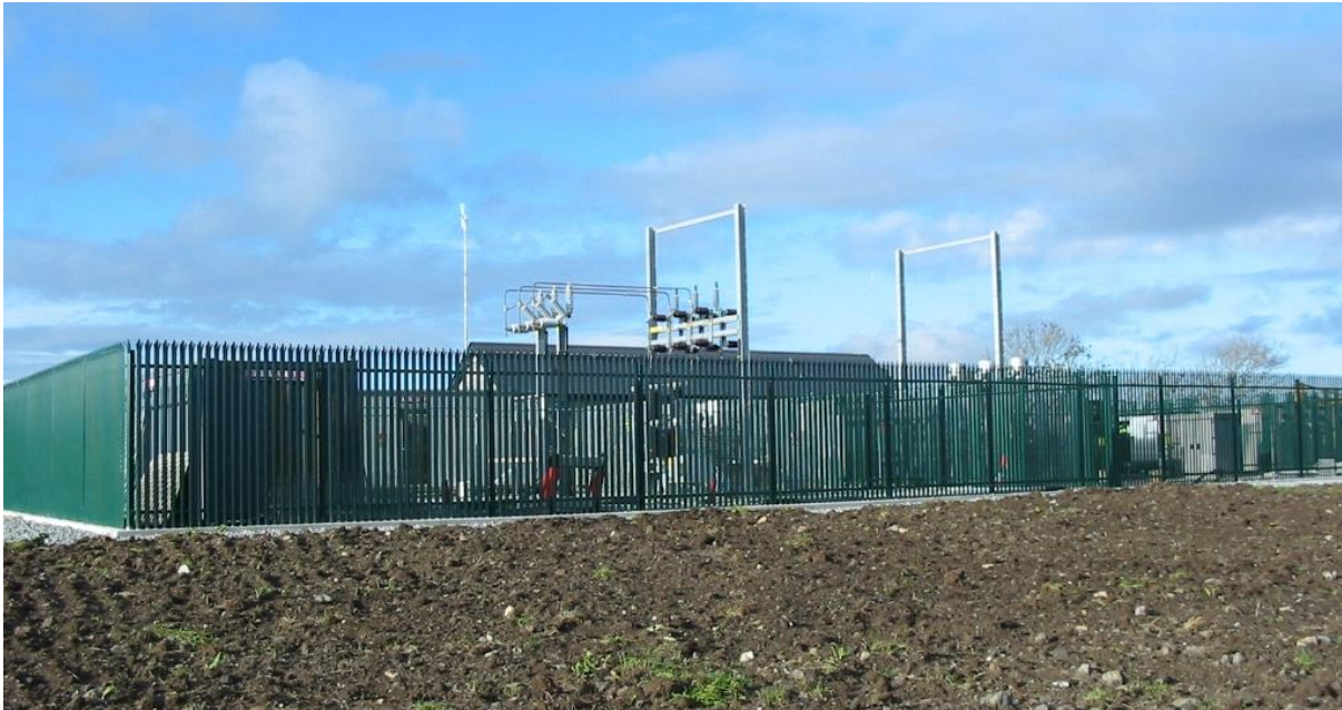
Figure 30: Typical Substation Compound
