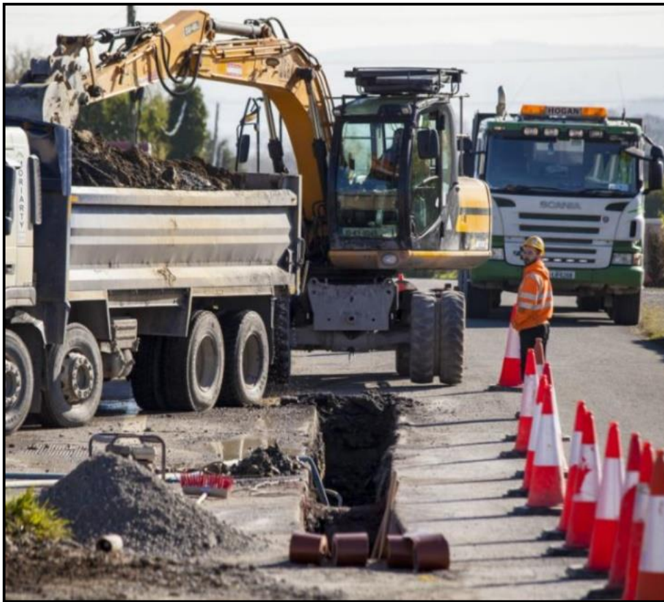
Figure 4-17 Typical excavation works for a grid connection cable trench on public road
