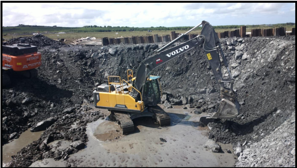
Figure 14: General Excavation towards the centre after fill is placed beside the sheet piles
