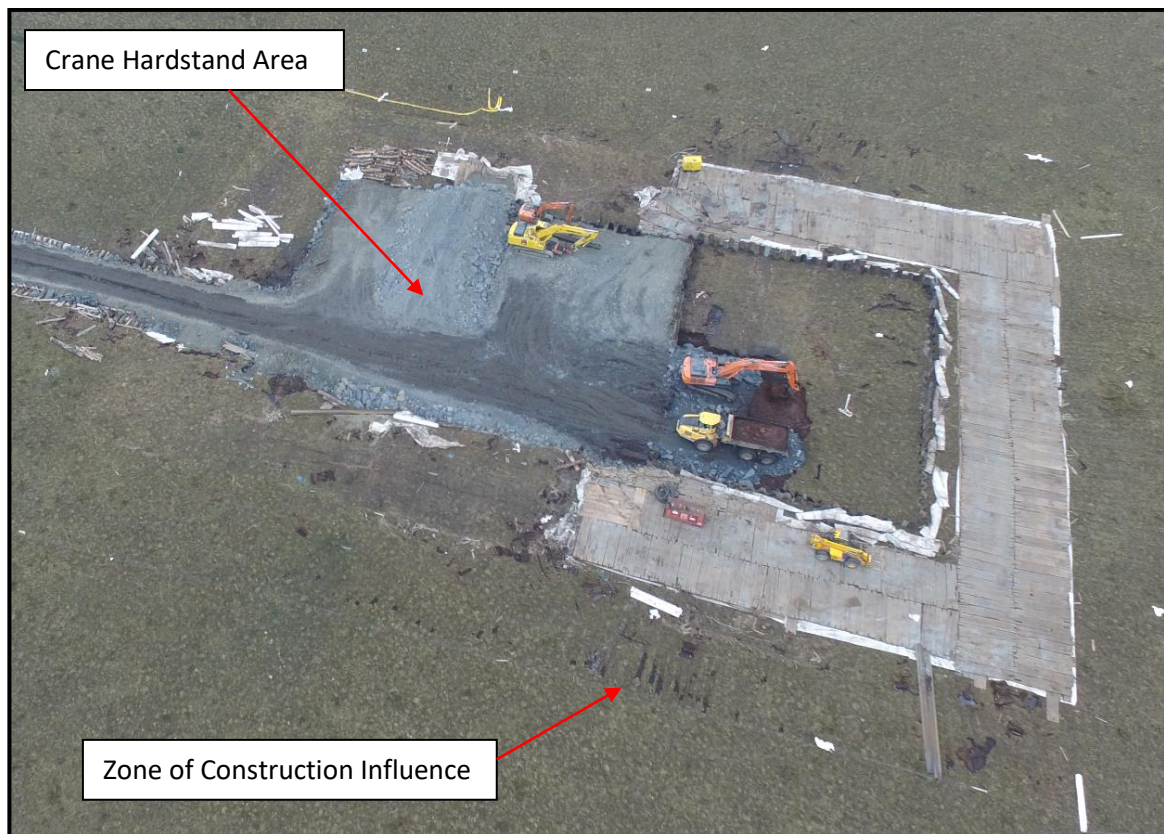
Figure 4-8 Photo of typical zone of construction influence around a hardstand in deep peat
